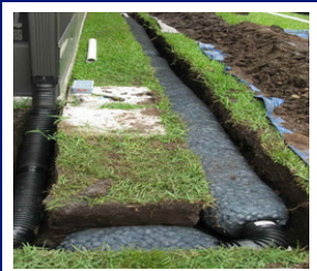
Downspout connected to a French drain; source: prosprinkler.com
